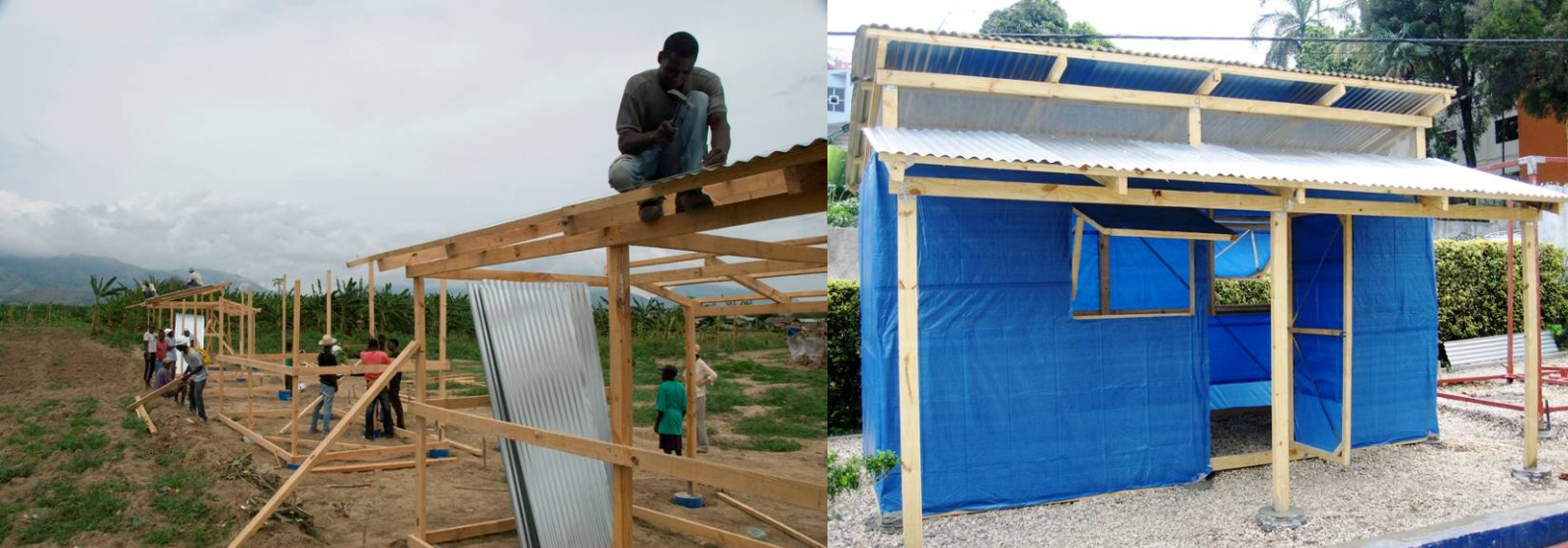
Left: Local professionals help build T-Shelters that are robust enough to withstand hurricanes. Right: A typical Habitat for Humanity T-Shelter has good ventilation, mosquito nets, a strong frame with cross bracing, and either permanent concrete foundations or temporary concrete anchors so that the structure can be moved to a permanent site.
